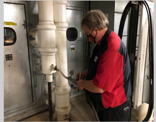
Maintenance Mechanic Wayne VanderArk performing chilled water startup procedures in Biochemical Sciences.
